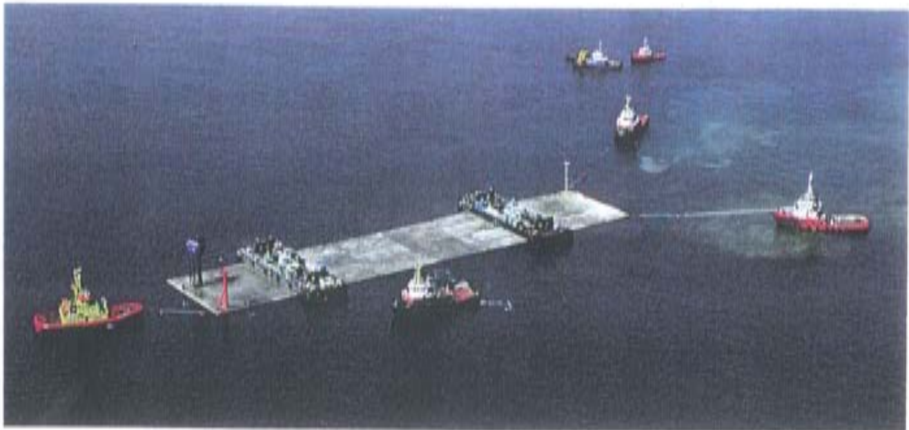
The first tunnel element is towed in the tunnel trench in Drogden.
